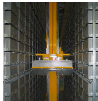
LASR—Library Automated Storage & Retrieval
